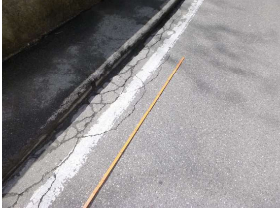
7524526_2016H_19-BELAG AM FAHRBANHRAND RISSIG
